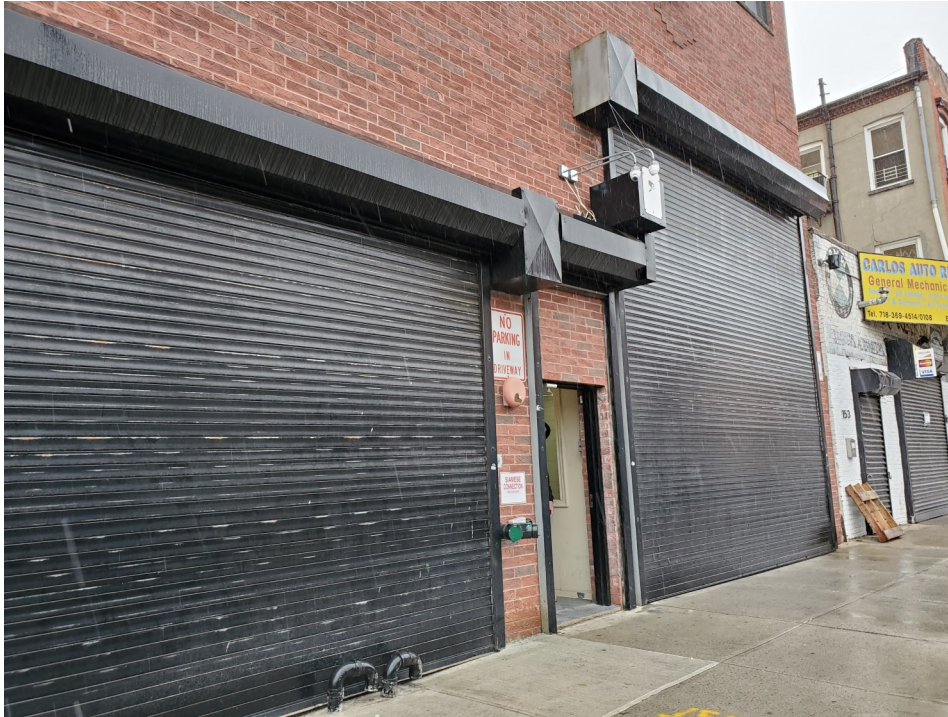
Photo 5: View of Garage Bay Doors on the Southern Side of the Site Building.
